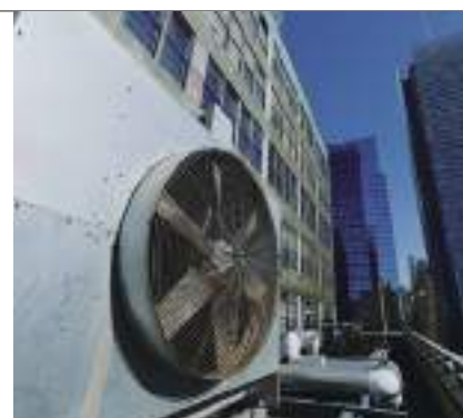
Air conditioning system
