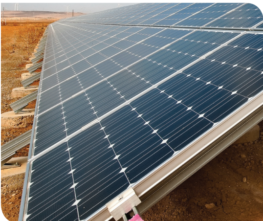
Photovoltaic power generation
